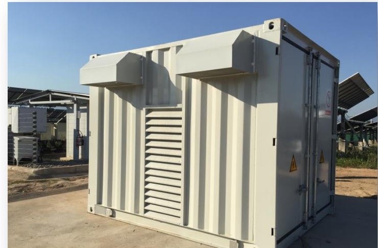
Demonstration set of 700 KWh battery with Solar system in Lampang
