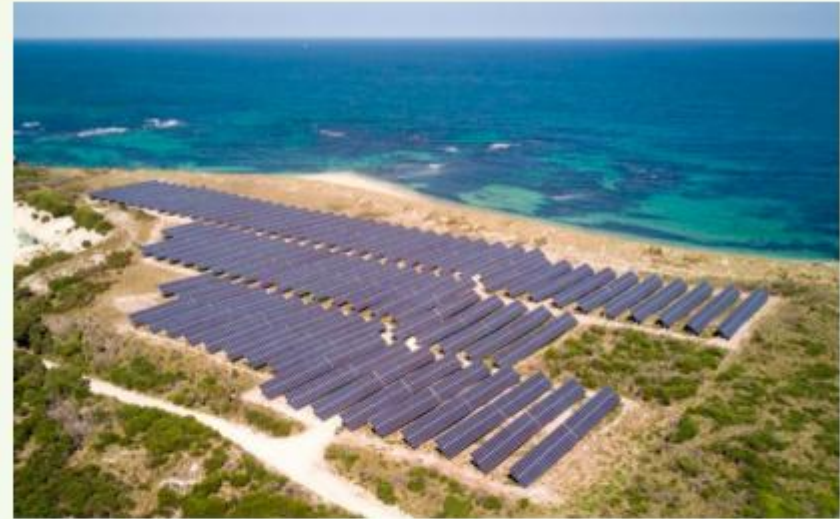
The Garden Island solar power plant. Source: Carnegie Clean Energy
